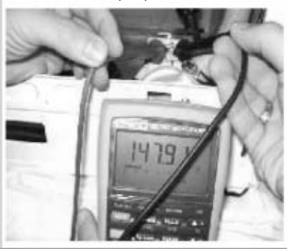
PICTURE F5-2: pump resistance is being measured over the pump connector
