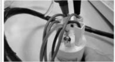
Picture F13-2: 220VAC control on U outlet ends of the noise filter
