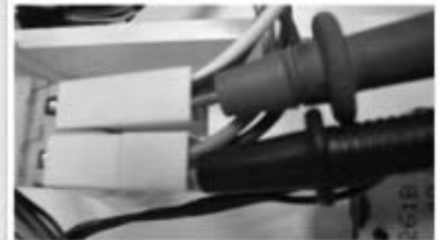
Picture F13-4: 220VAC control on outlet ends while On-off key is pressed
